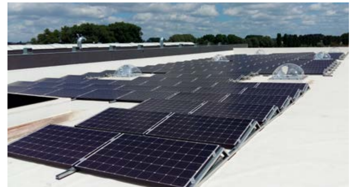
Roof insulation, Light Catchers and solar panels
